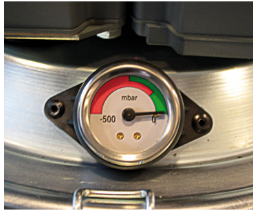
Filter Blockage Indicator Gage.
